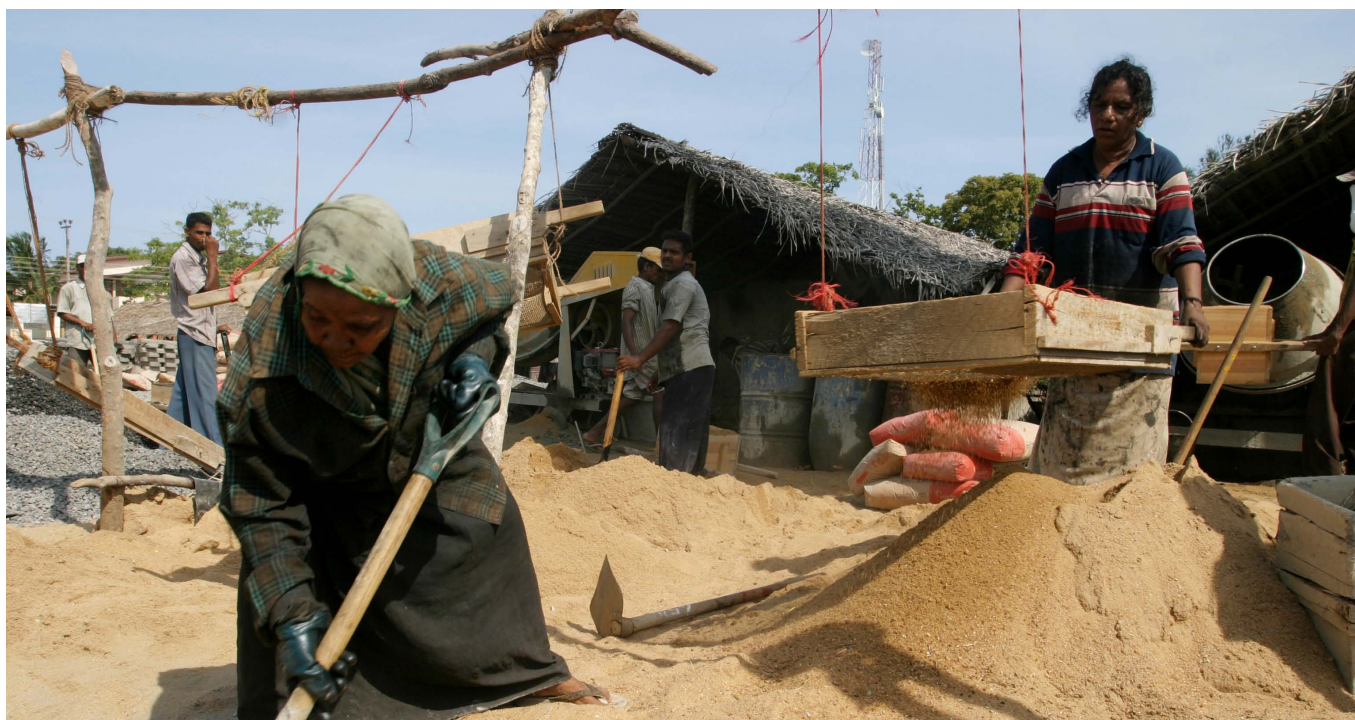
Capacity development of local suppliers, such as these brickmakers in Sri Lanka, should focus on building skills transferable to a post-aid business world.
